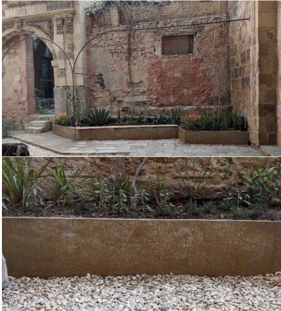
Figure 19: Rusting finishes of the steel [Source: Researchers]
