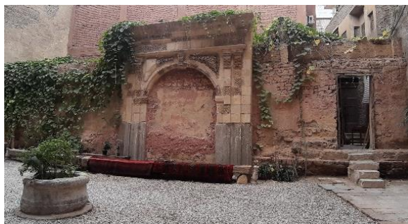
Figure 16: The initial old historical Gate condition, and the existing entrance and stairs. [Source: Researchers]
