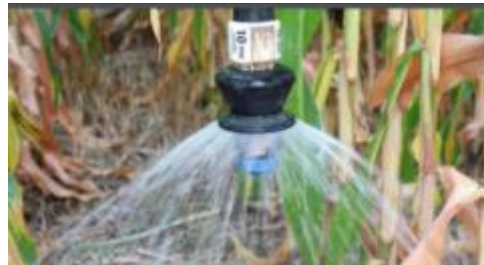
Fig. 5 - Low-pressure and rotating sprinklers
